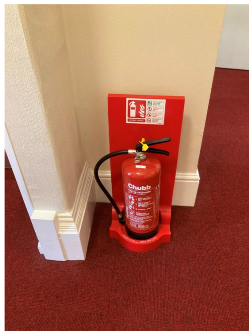
Identified Firefighting equipment
