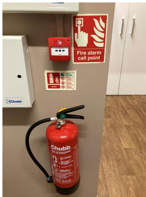
Woodhouse Identified Firefighting equipment
