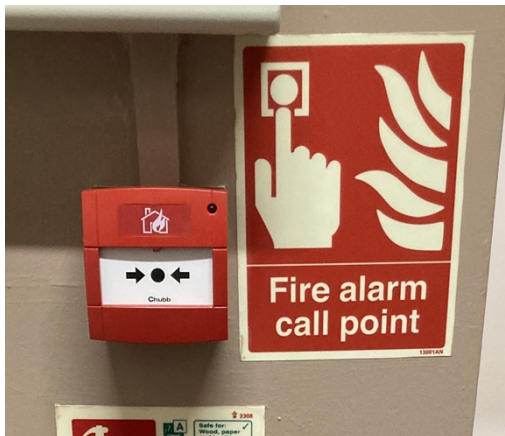
Woodhouse Identified Fire Alarm Activation Points
