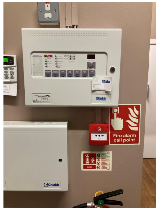
Woodhouse Fire Panel no faults displayed
