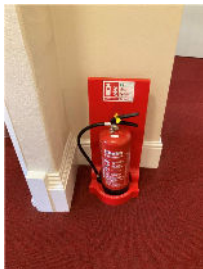
Identified Firefighting equipment
