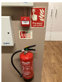
Woodhouse Identified Firefighting equipment
